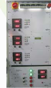
300kW Generator Control Panel
